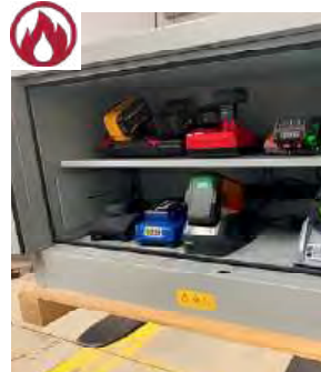
LITHIUM ION BATTERY CHARGING STORAGE CABINET PAGE 234
